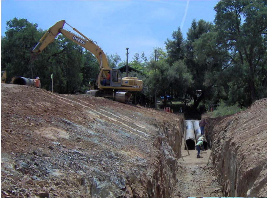
The photo at left and below depicts the contractor installing the revised design of twin 36" pipes to handle the required flow capacity of 35 cubic feet per second.
