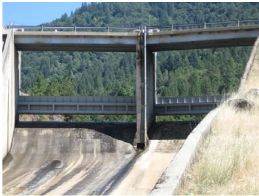
Opening Spill gates at Ponderosa Dam
