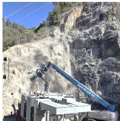
Figure 2.) Hillside post installation of shotcrete on the NW face and rock netting on the NE face
