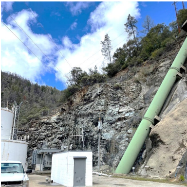
Figure 1.) Hillside above WPH Transformer 2023
